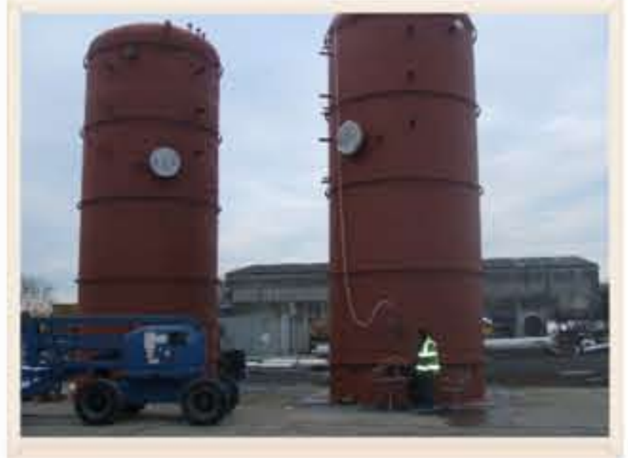
Two off 140mtr 3 -PD5500 Cat 2- Carbon Steel Thermal Stores being hydrotested in yard, prior to being insulated and clad inside workshop.
